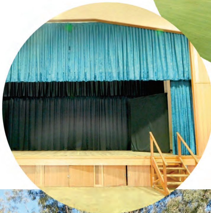
Photo below right: New fire proof stage curtaining installed at the Barellan Community Hall.
