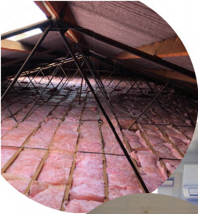
Photo left: Ceiling insulation within the Grong Grong Commemorative Hall and School of Arts.
