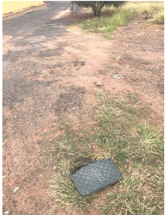
Photo 18: view of site water connection at Watkins Lane
